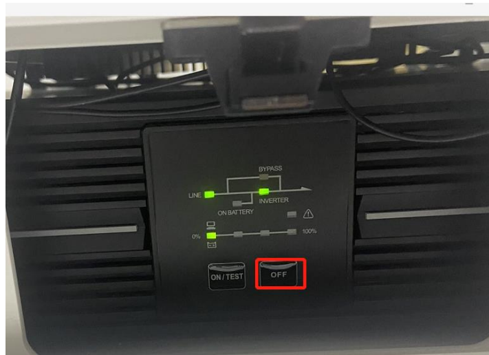
Figure 4. 5 Operation panel of UPS power supply.
